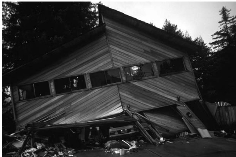
Loma Prieta, California, Earthquake October 17, 1989. Boulder Creek in the Santa Cruz Mountains. The lack of adequate shear walls and construction on fill contributed to the failure of this structure. U.S. Geological Survey
